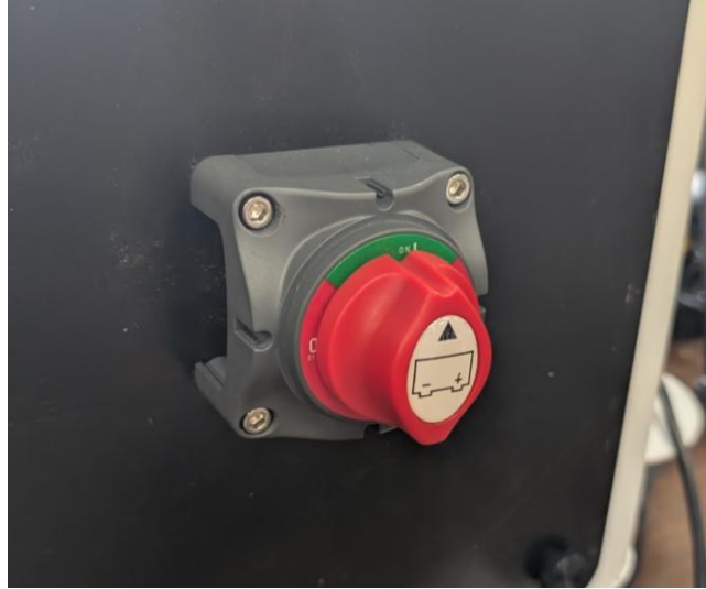
Figure 36: Charging station emergency circuit breaker switch
