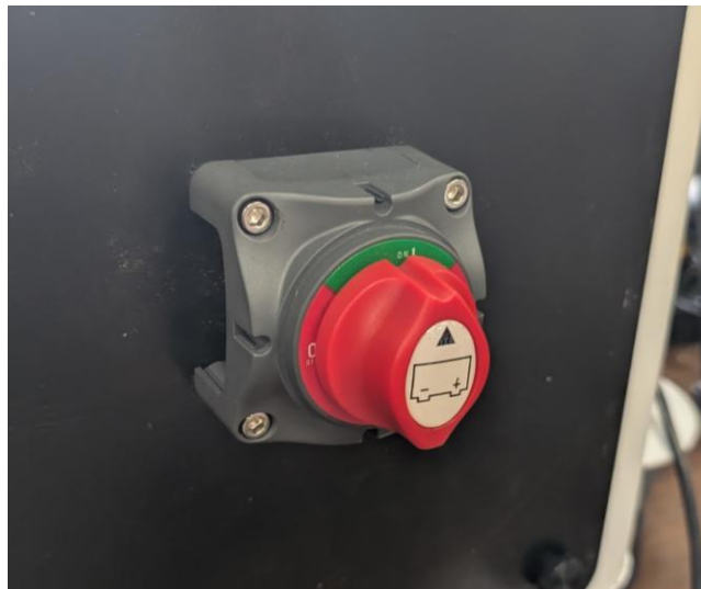
Figure 4: Charging station emergency circuit breaker switch
